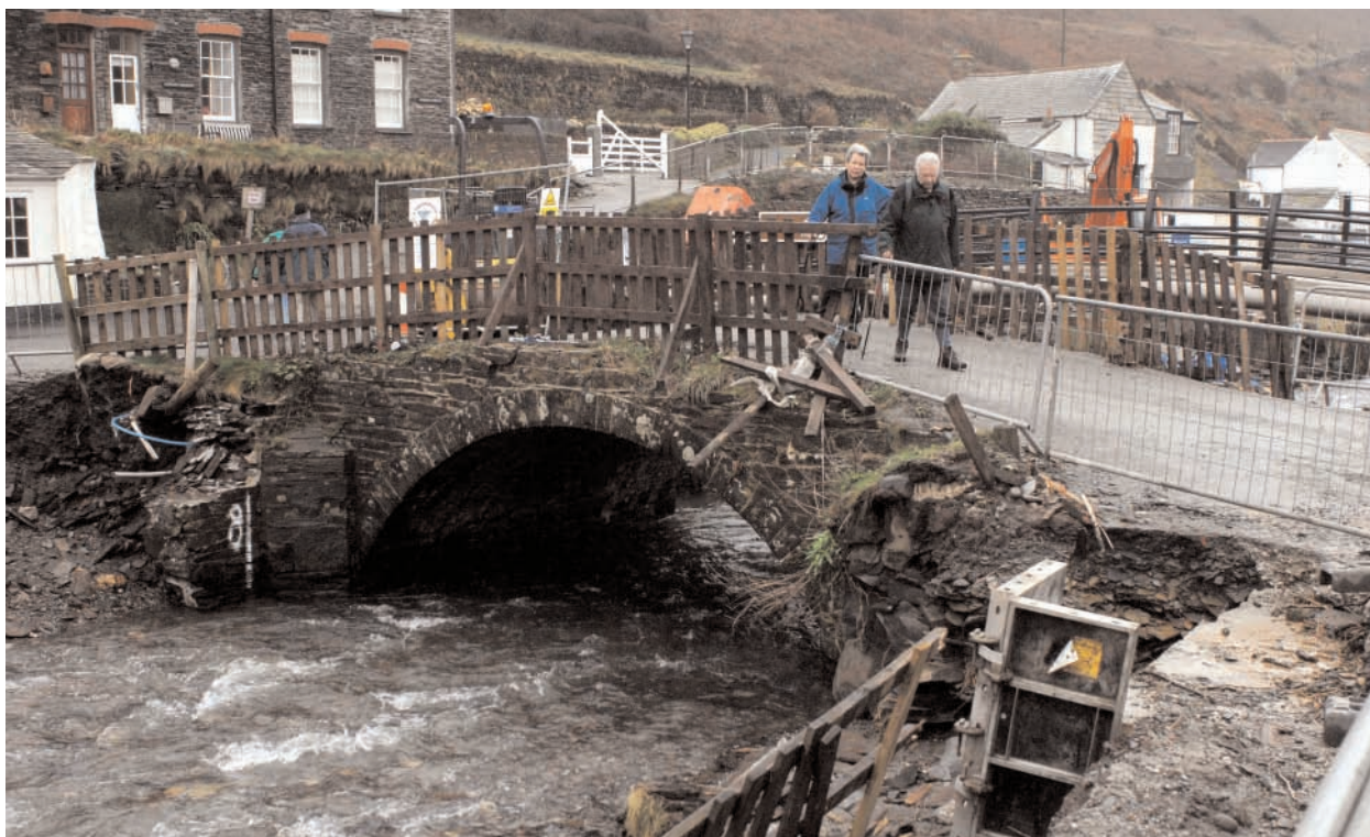
Old and new: The old Lower Bridge is about to be removed to reduce flood risk in Boscastle – its new replacement can be seen behind it with the handrails in place
